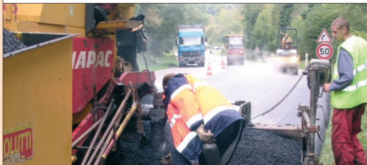
Integration of the SURE process into the maintenance programme: case of the RN 138 pilot site in the Eure region between Bernay and Saint-Denis-Des-Monts.
